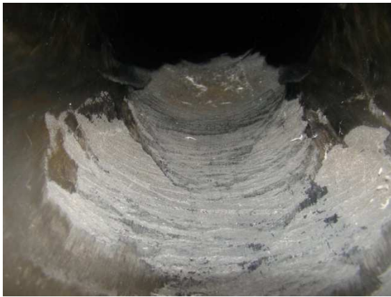
Fig. 1: Defective barrel showing sintered sand particles
